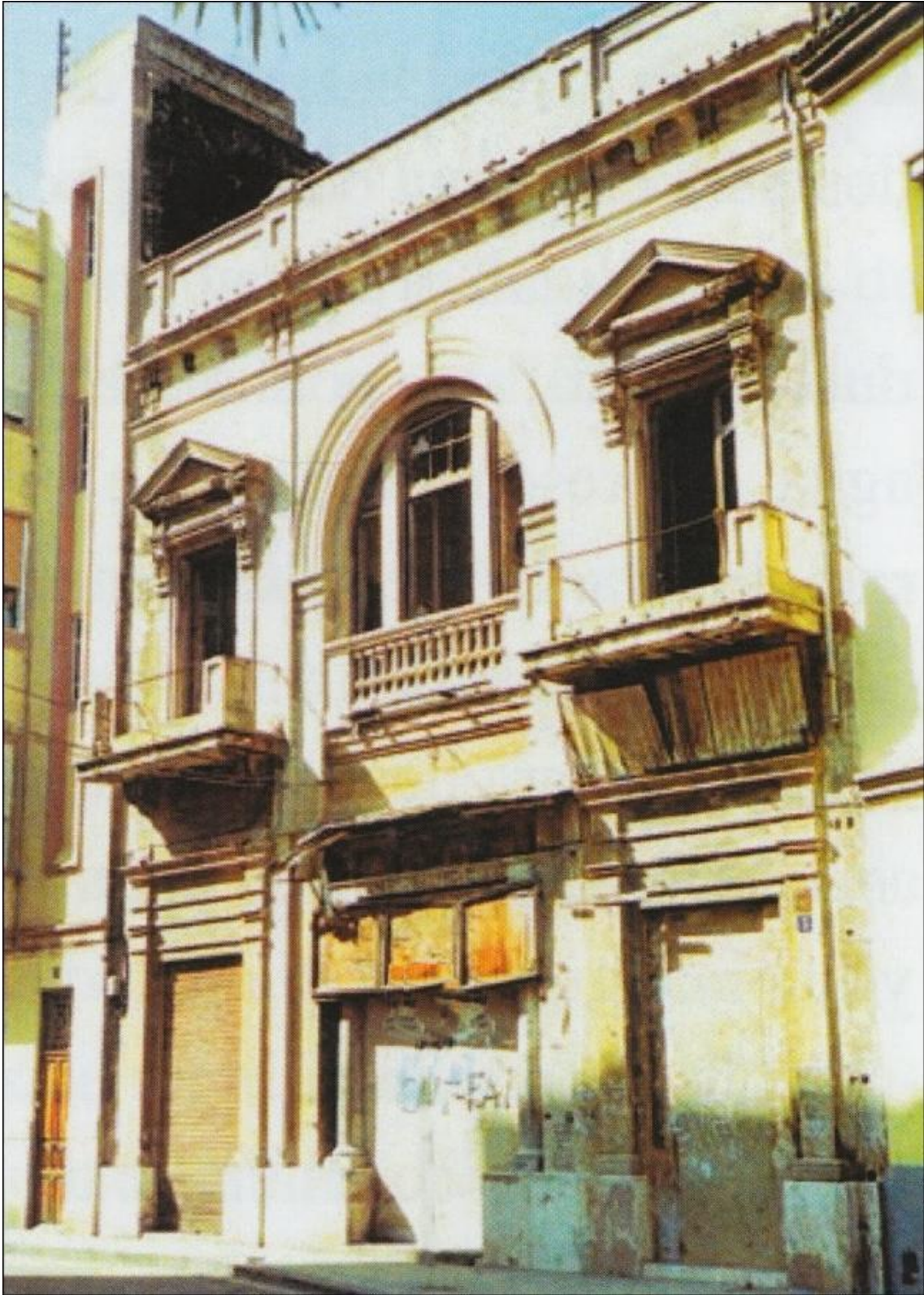
The theatre in a state of neglect.
